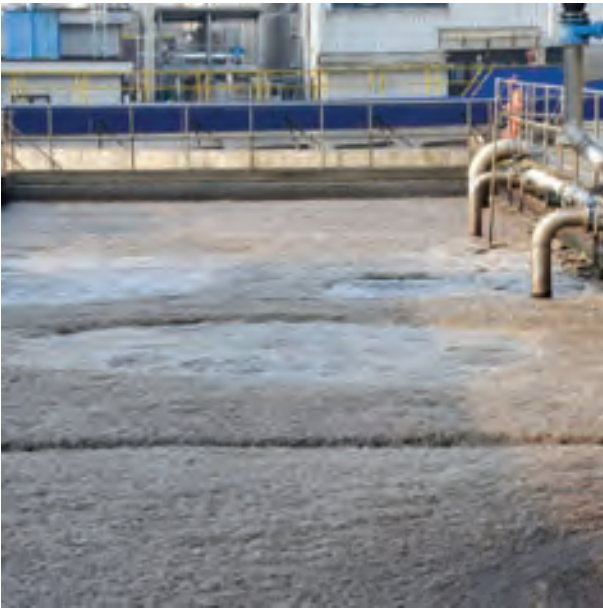
Sludge treatment and disposal
